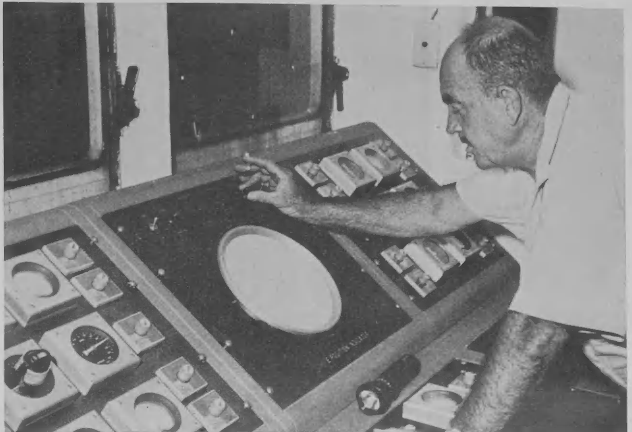
THE CONTROL center of the automatic positioning equipment aboard the floating drill rig Caldrill I is this control board which computerizes four
